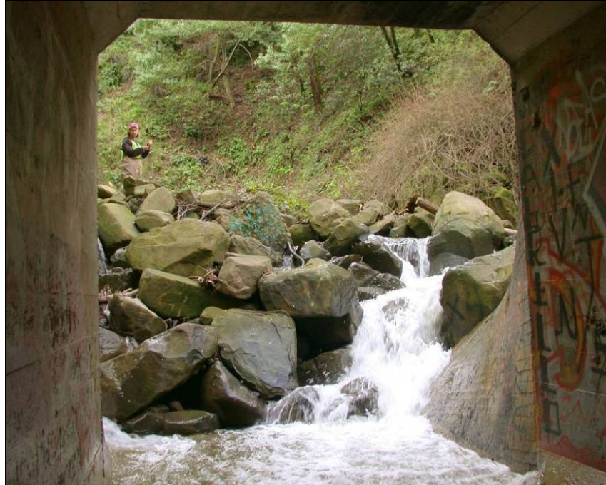
Figure 2.2 - Inlet of the downstream crossing (MP 8.75), as flow cascades down a 5.5 foot drop over boulders deposited due to the channel constriction caused by the culvert.
